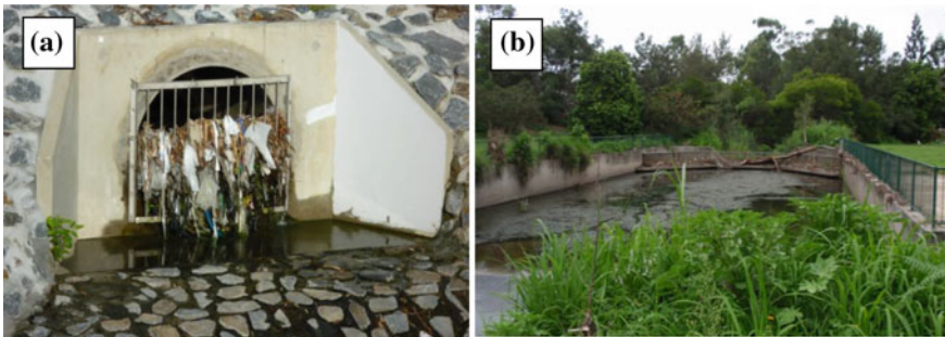
Fig. 1.2 Typical GPT devices. a Trash rack. b In-line screen
